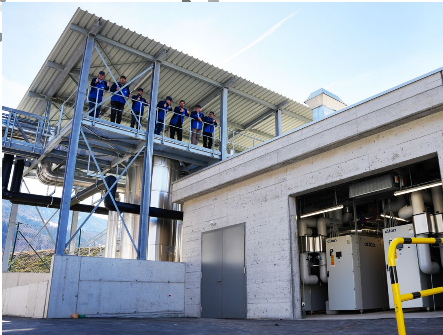
Newly installed heat pumps at Grünenthal's API site in Mitlödi, Switzerland
